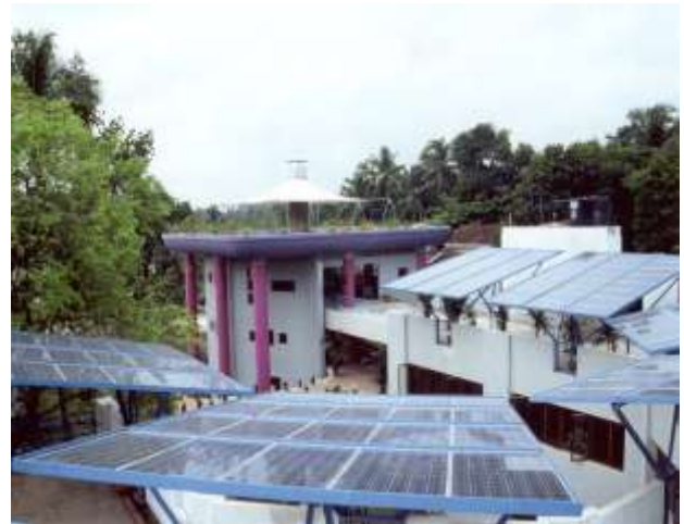
Solar PV modules replace traditional roofs as shade and water catchers. Large overhangs stop the blazing sun from reaching the building walls. White tent like structures are used as shades, and more are being installed now. Large ducts, extending above the tents, extract air from the rooms to cool the building interior by a natural ventilation system which is assisted by solar PV driven fans. In addition to this vertical ventilation and cooling, horizontal cross ventilation is extensively used.
